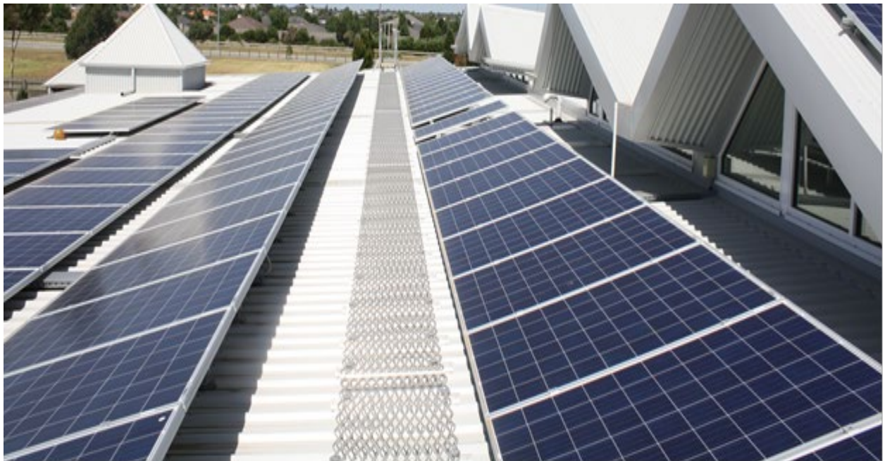
Image 5: Arena Family and Child Centre Solar Electricity System
